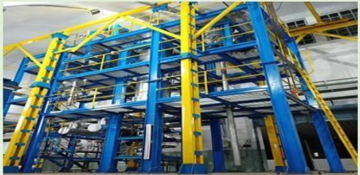
Fluidized Bed Gasification Pilot Plant
